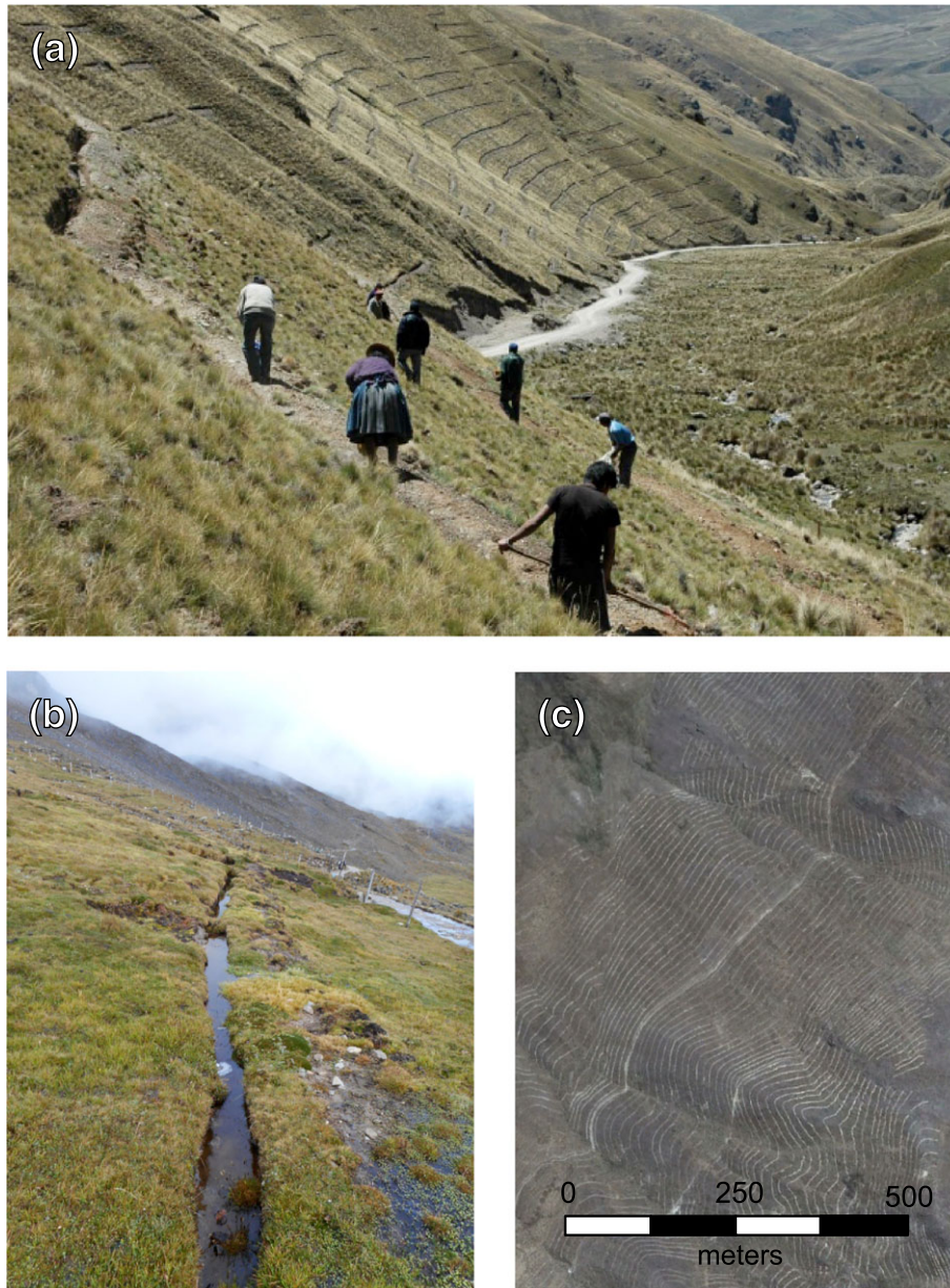
FIGURE 2 (a) Construction of infiltration trenches as part of the World Bank- and CARE-funded PRAA project. Photo taken from Comunidad Andina presentation. (b) Infiltration trench with ponded water. (c) Aerial view of trenched hillslope in the Shullcas Watershed, from Google Earth™
